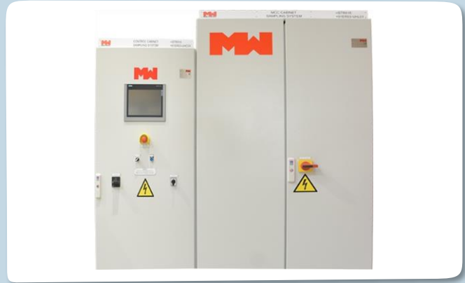
Control Cabinet – Central
