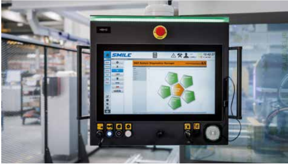
Operating panel (HMI)
