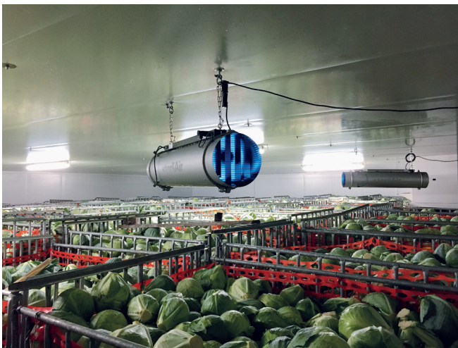
pic 2 3 : sterilAir UVR-4K Air disinfection unit in a vegetable storage room
