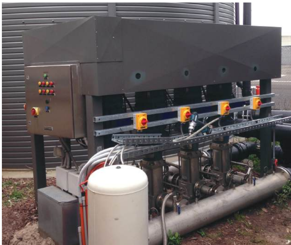
KATKO EMC safety switches installed to a water purification system at the Sydney International Airport.
