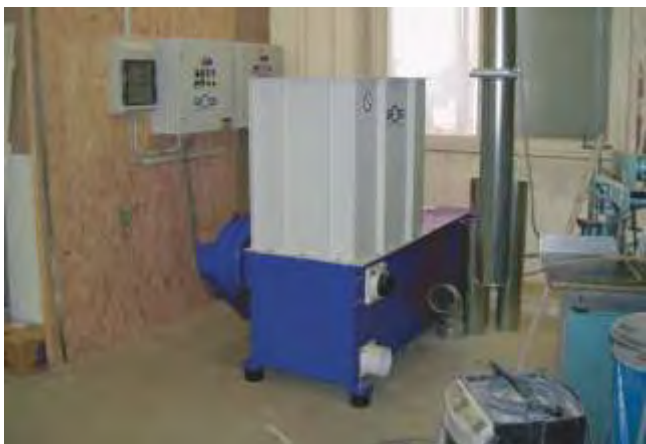
GAZ 62 shredder connected to an air suction system
