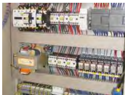
Switching cabinet / SPS control
