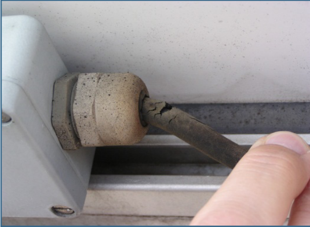
Cable overheating effect
