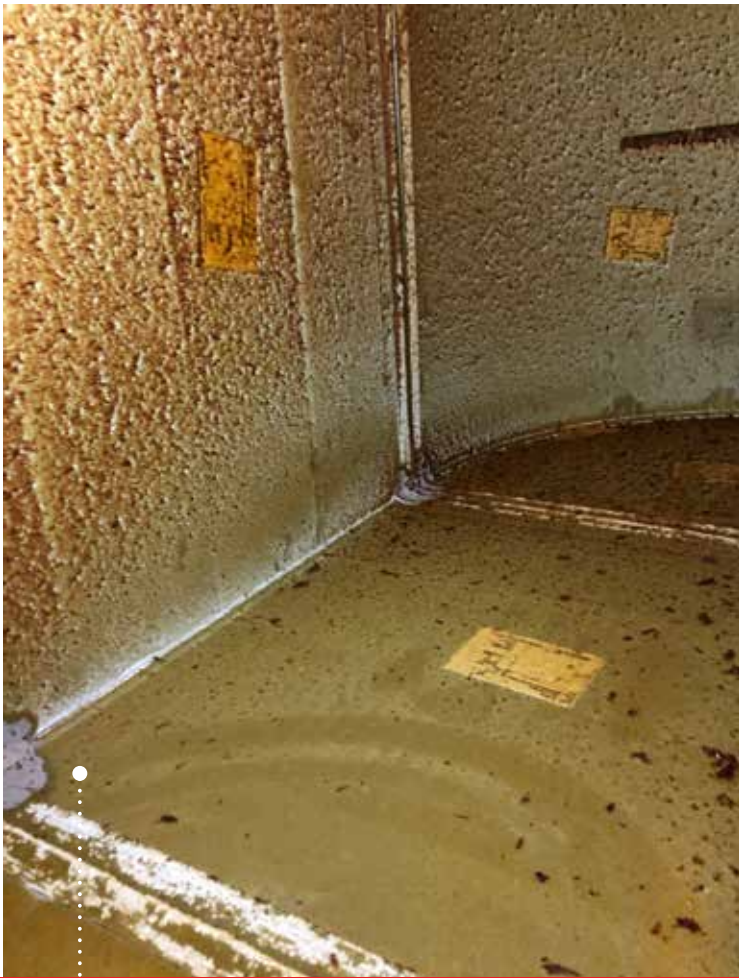
Grill duct with JIMCO Technology - Not cleaned for 60 months
