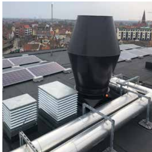
Air outlet from the kitchen
