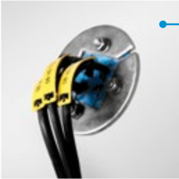
Air lock room: Sealing of communication and signal cables for CCTV, computers and security equipment in panel wall.
