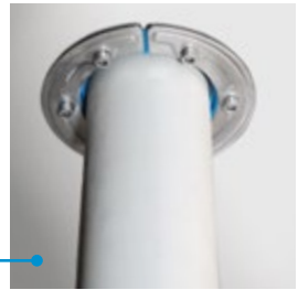
Above glove box: Roxtec RS seals and sleeves are used for sealing extract ducts through ceiling.
