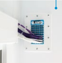
Bio safety laboratory: A powder coated easy-to-clean Roxtec frame sealing a wall transit.
