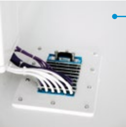
Corridors/lobby: Power and lighting cables sealed by the Roxtec cleanroom frame.
