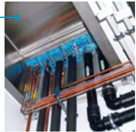
Pipe inlets: Sealing of various pipes bringing water and medical gases into the room.
