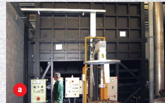
Silo polmone / Storage bin
