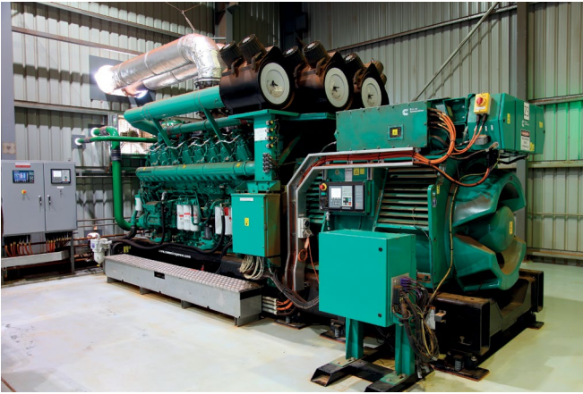
One unit of the QSK95 Series generator set (C3500D5) installed at Cloudbreak Mine delivers 3,125kVA of reliable prime power.
