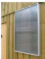
Solar collector panel on the exterior wall of a holiday home
