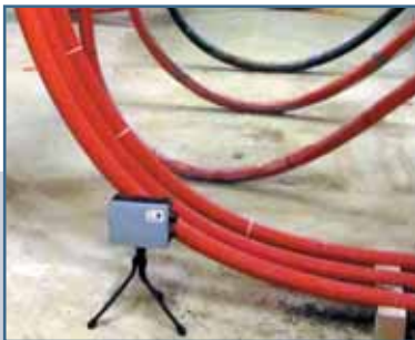
On power cables
