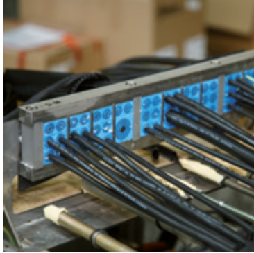
Driver cab and engine room: Customized sealing solution installed to keep tight between the driver cab and engine room.
