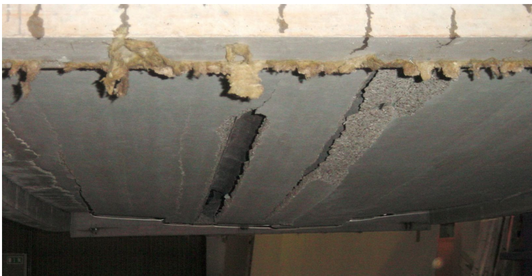
Figure 2. Damages after 25 minutes standard fire on two extruded hollow-core slabs with cast groove between and cast into a reinforced frame. Test from 2004 (H138 in [2]). Photo K. Hertz.
