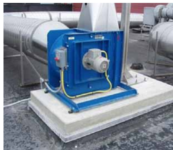
Fan placed on the roof.
