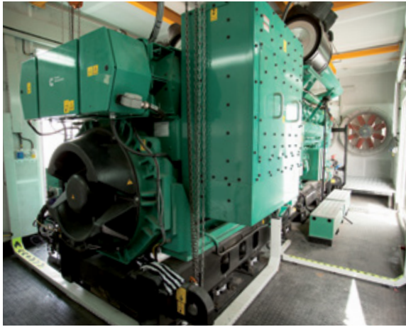
SEC added a QSK95 Series unit to its existing generator set array
