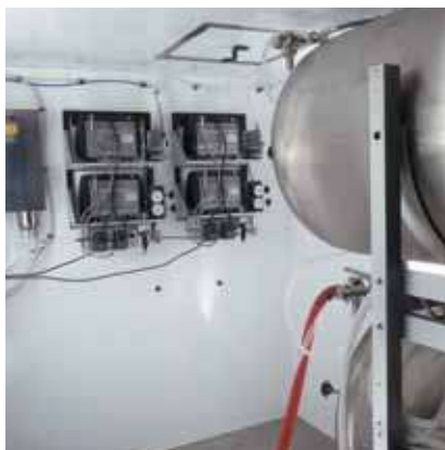
Compressors used for beverage dispensing
