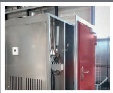
The redundant air conditioning module ensures that the ValueShelter is always kept cool.
