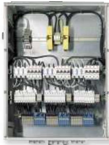
DC combiner box
