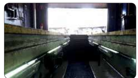
Example of LINE LIGHT 6 solution mounted in a truck mechanic's pit
