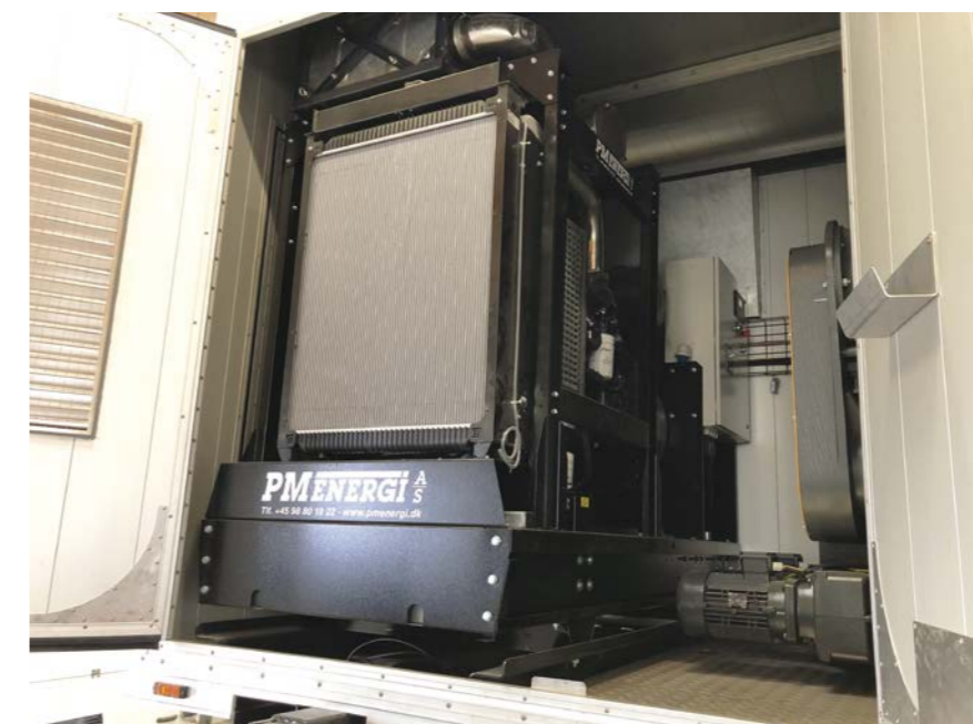
Engine room with diesel generator set and hydraulic station.
