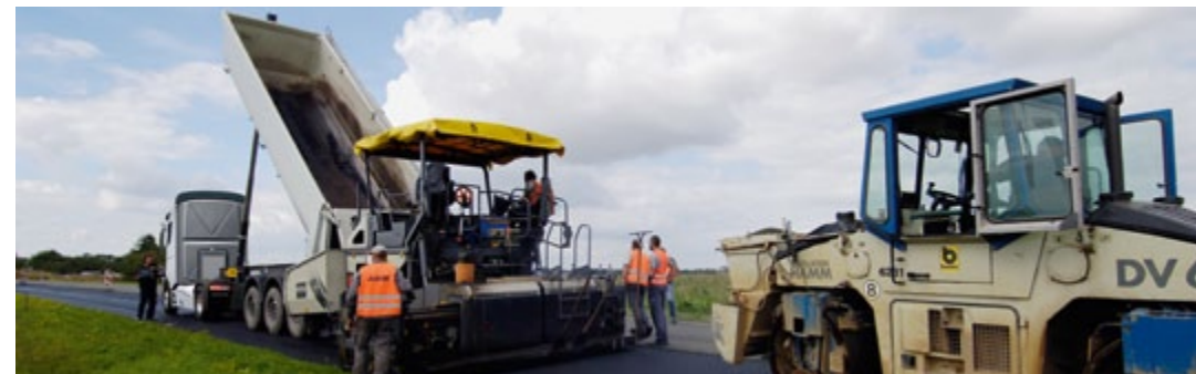
Tipper trailer with rounded steel body in use in front of the road paver.
