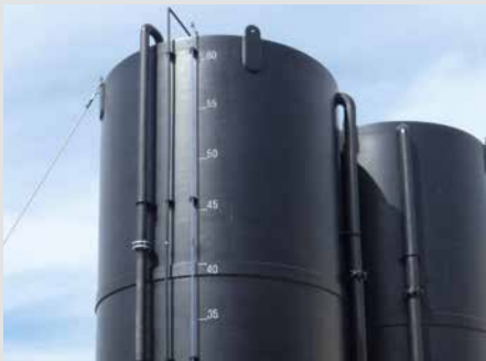
Storage tanks made of polyethylene
