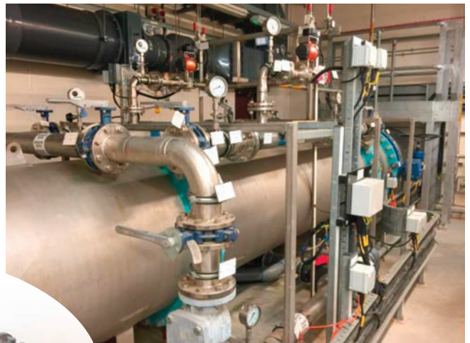
GDS installed at customer site
