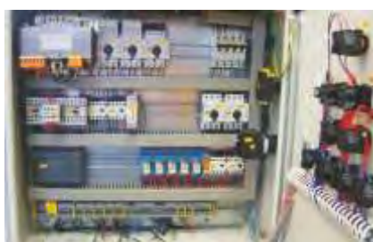
PLC controls / control cabinet
