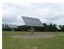
Grid connected PV tracker Plant
