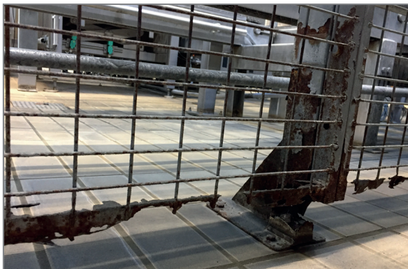
In the food processing industry, guarding solutions in corroded conditions like this, are unfortunately still seen.
