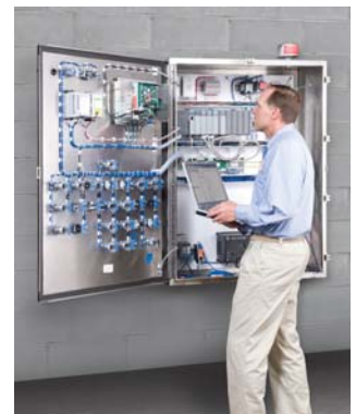
Plant personnel can download programmes to start, stop, slow, speed-up, delay, advance or cycle equipment functions.
