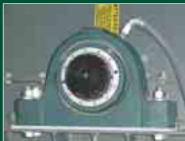
Bearing temperature sensor on belt conveyor
